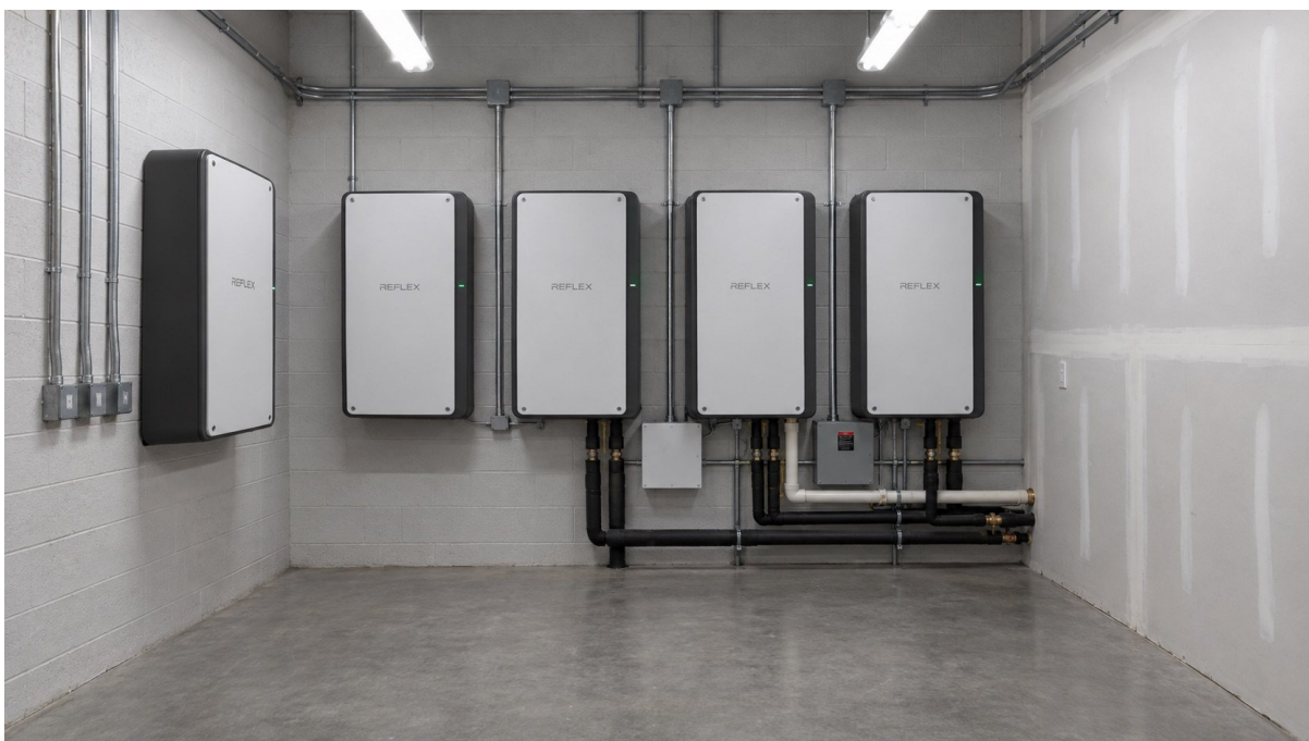
Figure 3. Liquid-cooled nodes in a plant room. Nodes mount on the wall and connect to the building loop; no raised floor or data hall.
